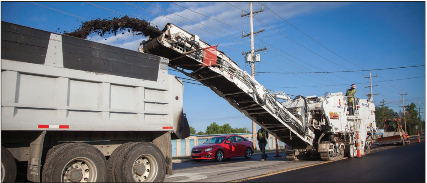
The Roadtec RX-700e Cold Planer is a heavy-duty milling machine, well suited to projects requiring cut depths of up to 14". Fittingly pictured outside Millville, Ohio, Welfle Milling Foreman Bobby Beese and his crew work south on Rt. 27.
