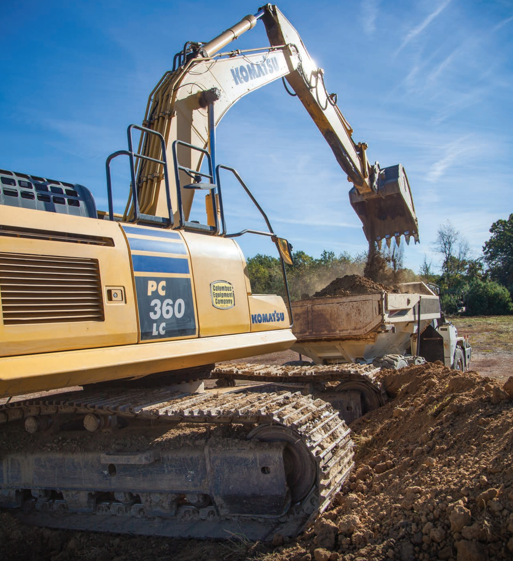
Luburgh's 25-year veteran Operator Brian Barker on a private site development project in Norwich, Ohio with a Komatsu PC360LC—one of almost 40 hydraulic excavators the company now owns.
