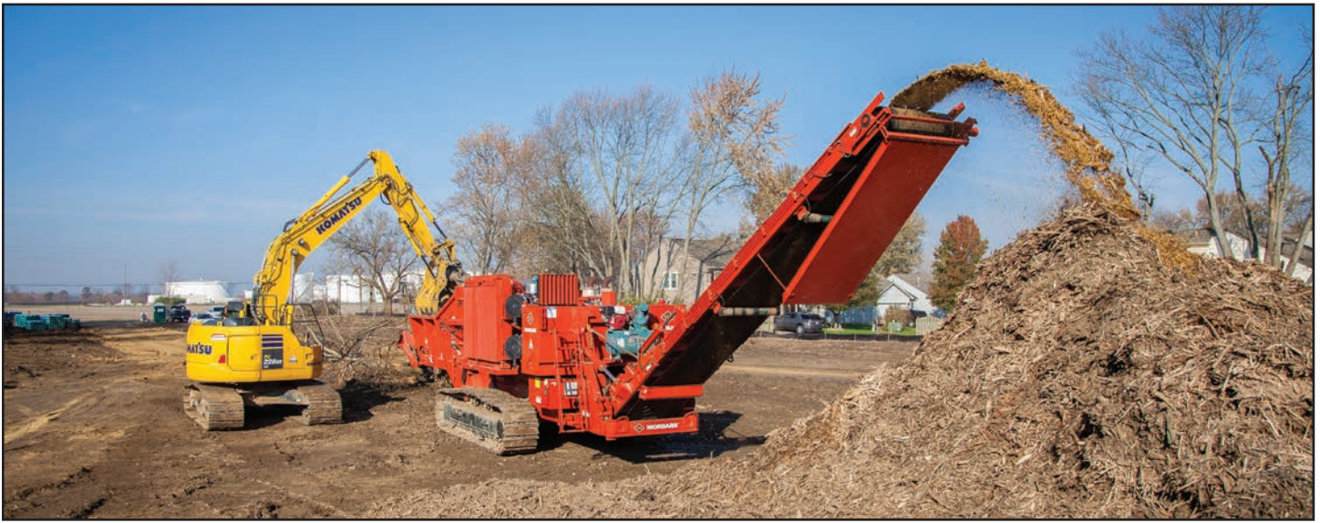
The Snider Group's Morbark 6600T Wood Hog Horizontal Grinder has been an excellent fit for the land-clearing work the company performs. The 6600T is pictured clearing seven acres of woods on the Tansel Crossing Subdivision Project, Section 1, in Clermont Indiana, just west of Indianapolis.
