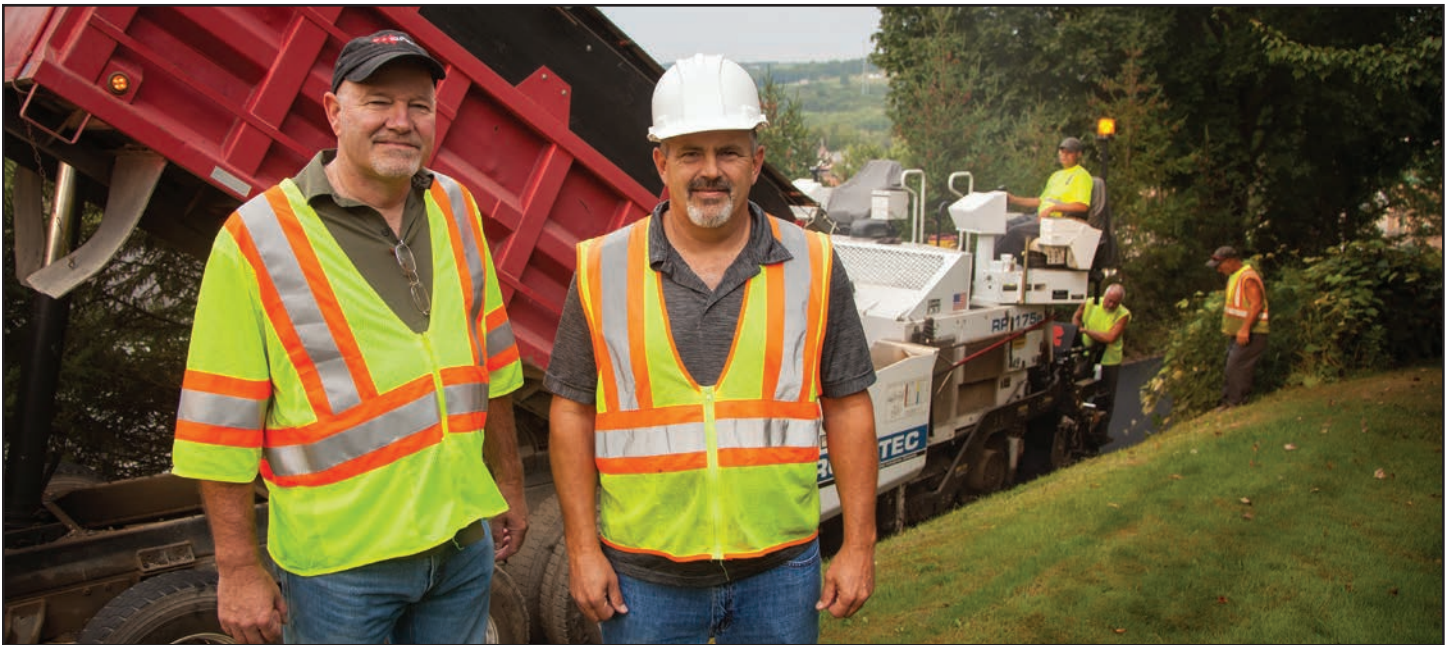
Melway Paving Vice President Phil Schlabach (left) and Estimator Terry Triner pictured just north of Liberty Street, in the hills above Millersburg, the county seat of Holmes County, Ohio. The company has relied upon dependable Roadtec pavers for 15 trouble-free years.
