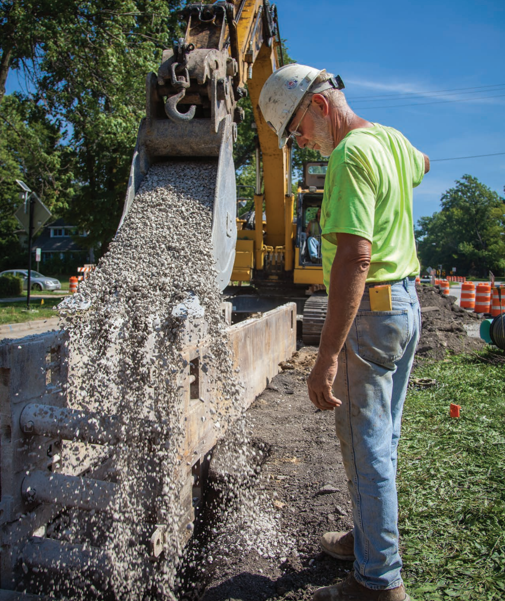
Fabrizi Site Foreman Larry Norman (foreground), Operator Jeremy Boudinot and a Komatsu PC228USLC excavator work together, balancing power and precision, on a sewer replacement project on Fairmount Boulevard in Cleveland Heights.
