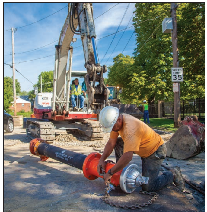
Laborer Joe Minarchek and Takeuchi TB290 Operator Mark Deanna prepare a fire hydrant for installation on Wooster Road, Rocky River.
