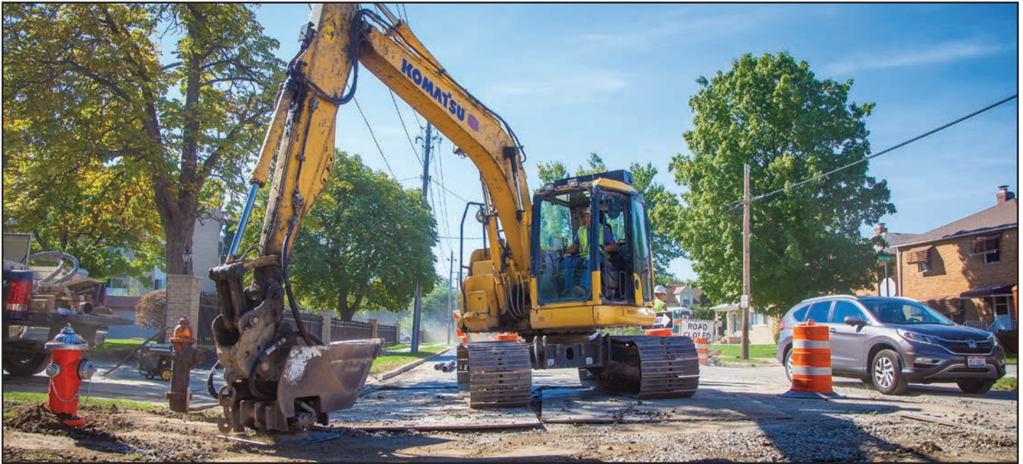
Komatsu equipment is popular with both Fabrizi operators and Fabrizi management. A PC228USLC excavator is seen here on a $1-million Wooster Road project—encompassing 6,662 linear feet of water main replacement to both high- and low-pressure service zones—in Rocky River.
