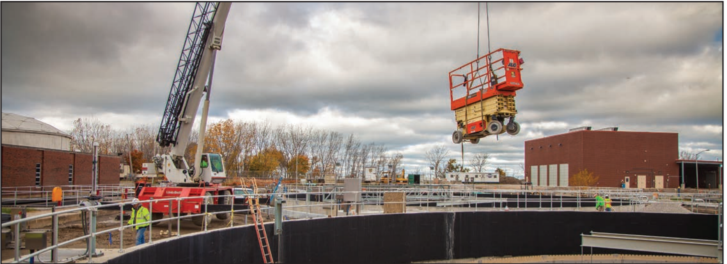
Shook's Link-Belt RTC-8065 Operator Joe Carlone relocates a 4,500 lb. scissor lift at the Easterly Waste Water Treatment Plant in Cleveland, Ohio. The 8065 is rarely idle and has seen over 6,000 hours of action in less than four years at the facility. Easterly serves over 334,000 residents and businesses, treating more than 94 million gallons of wastewater per day.
