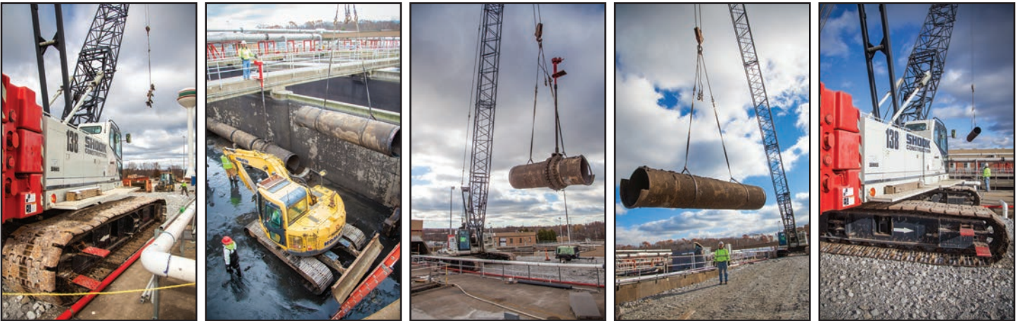
Shook Construction Foreman John Kunkler, Operator Curt Shepler and crew onsite at the Canton Water Reclamation Facility. The $81 million project is one of the largest public works projects in Stark County history. Upon completion, Canton will have the biggest wastewater treatment facility using membrane bioreactor technology in North America.
