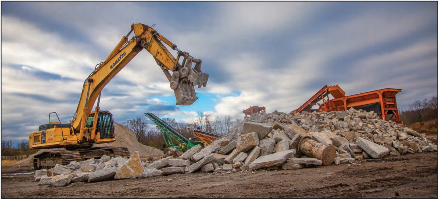
Charles Jergens' Eagle Crusher 1200 CC crushing and screening plant recycles internal and third-party, demolition material into 304. According to President Phil Jergens, approximately 80% of the company's customers use the clean, concrete 304 product due to the significant cost savings—often around 40%—over limestone 304.
