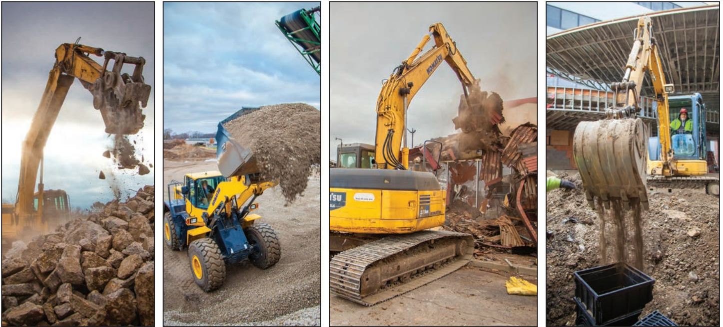
Whether it's material processing and handling (left two images above), demolition—PC228USLC Operator Randy Himes at a Miami Valley Hospital expansion site on Main and Stewart in Dayton—or site development—Ron Golub with a compact Komatsu PC35MR on a Dayton Children's Hospital development project—Komatsu equipment performance is dependable and unmatched.
