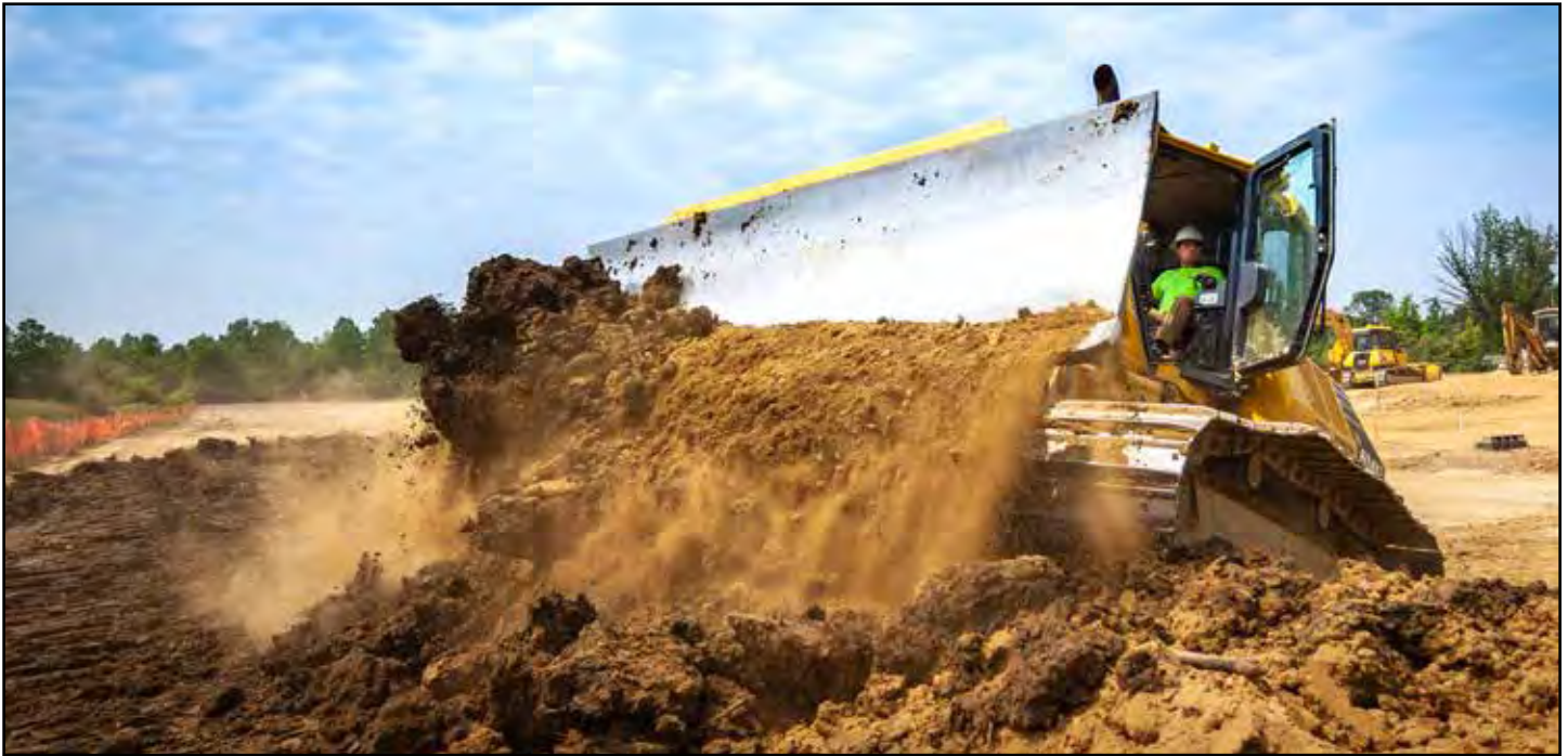
Fabrizi's Komatsu D61PXi is just one example of Komatsu iMC equipment that has brought speed, agility and efficiency to the company's operations. The workhorse is seen here on a $4-million project—a Lakes of Orange LLC residential development—in the Village of Orange, Ohio.
