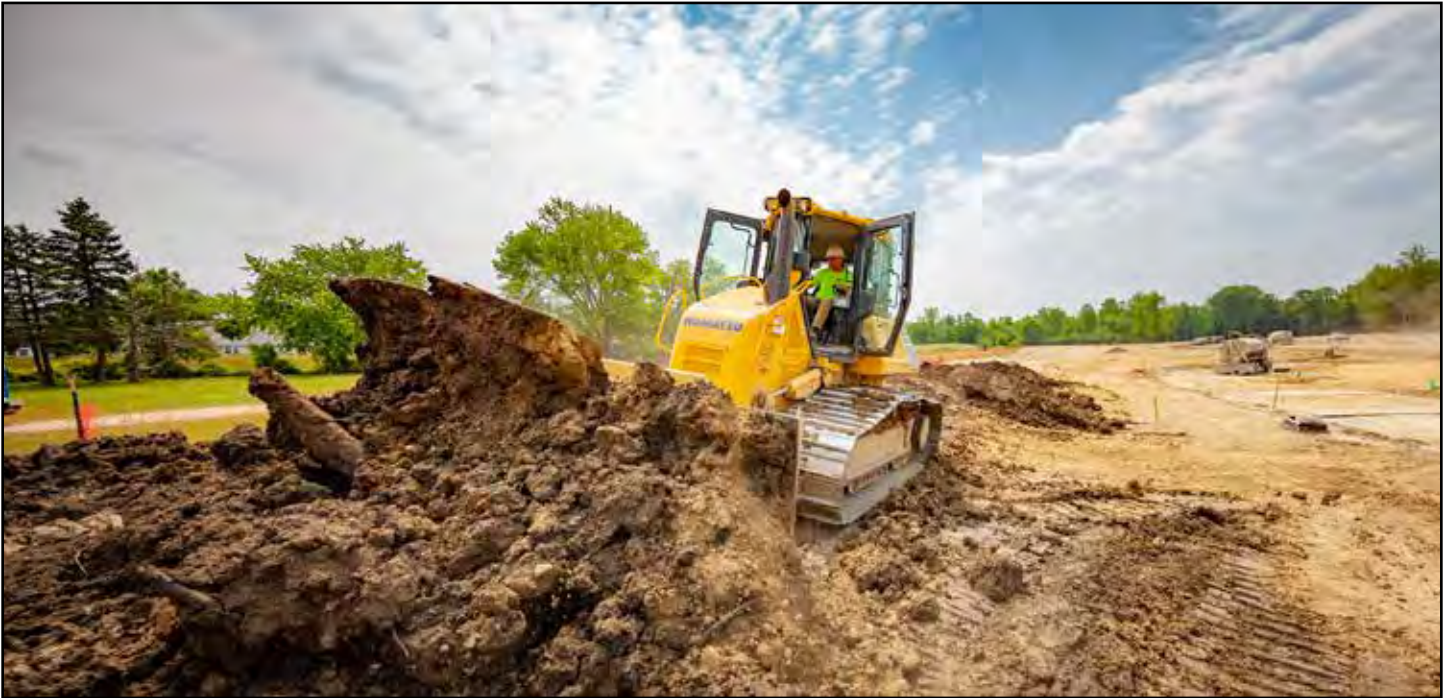
The Lakes of Orange development will offer more than 50 residential home sites, covering more than 20 acres. Fabrizi Trucking and Paving will move over 75,000 yards of dirt and install storm, sanitary and water utilities over the project's 9-month duration.
