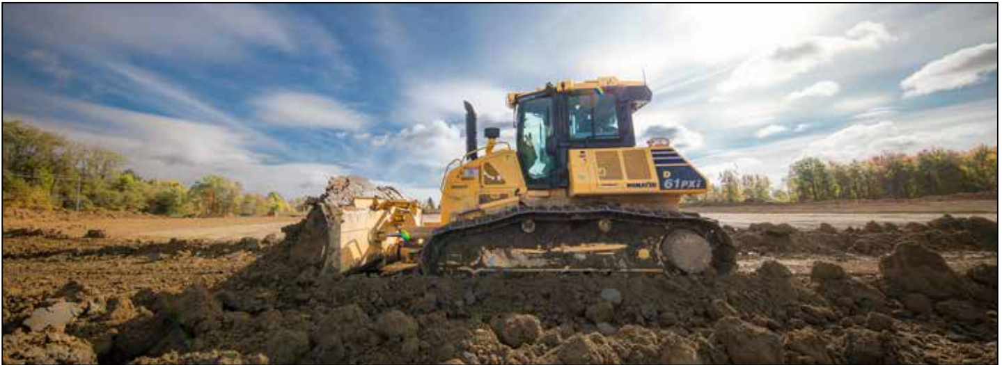
The Kufleitner project involves grading approx. 24,000 tons of aggregate base over a 55,000 square yard parking lot, approx. 4,000 feet of storm sewer, 2,000 feet of sanitary sewer and 1,600 feet of waterline. The Komatsu D61PXi handles it all in picture-perfect stride.
