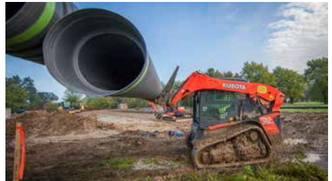
Operator Chad Seely moves storm pipe with the company’s Kubota SVL75-2 CTL on a commercial site development project in New Albany, OH.
