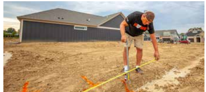
Foreman Jeff Combs marks dig lines at The Courtyards at Clear Creek development in Delaware, Ohio.
