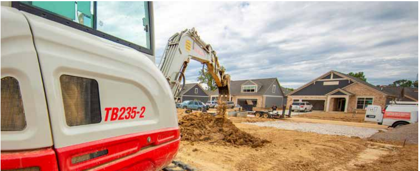
Eaton Plumbing Foreman Jeff Combs—seen opposite and above operating a Takeuchi TB235-2 excavator at Epcon Communities' The Courtyards at Clear Creek development north of Columbus, Ohio—has been with the company 12 years. From experience, he finds Takeuchi's power, comfort and versatility superior to competitive brands.
